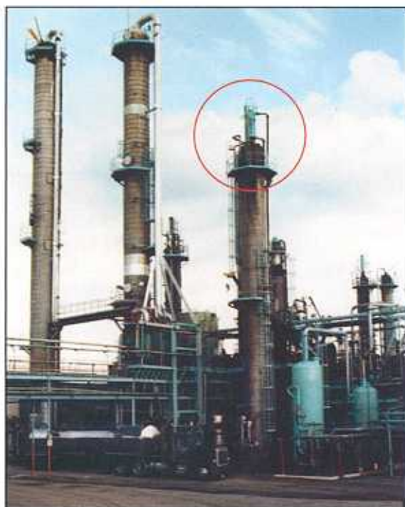
FIGURE 7. In this installation, a column-mounted spiral condenser is installed on top of a dehydrator column (and highlighted in the circle)
