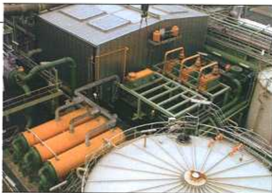
FIGURE 3. In this installation, three shell-and-tube (S&T) condensers are shown at the lower left, and three welded-block plate condensers are shown at the top right. Despite their small size, the block condensers have 50% greater capacity than the S&T units
